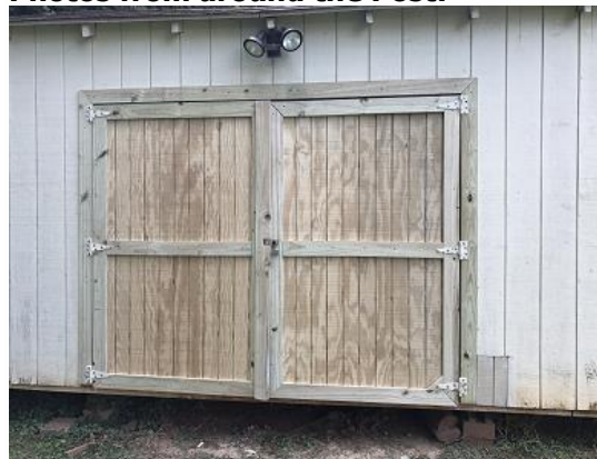
New doors built and installed by our member volunteers on the Post 72 shed
